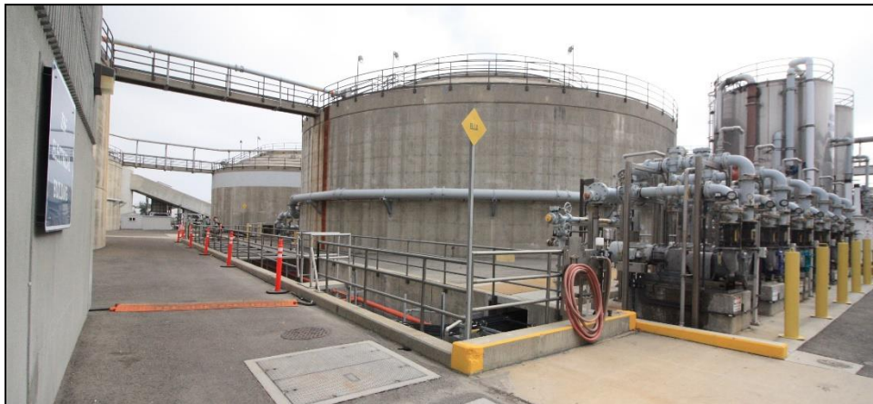
Orange County Sanitation District Plant No. 2 – 150626.00
