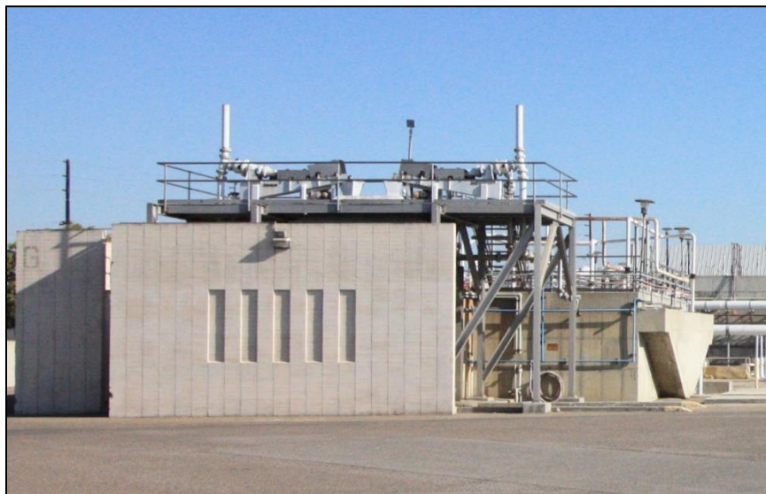
Orange County Sanitation District Plant No. 1 – 150626.00
