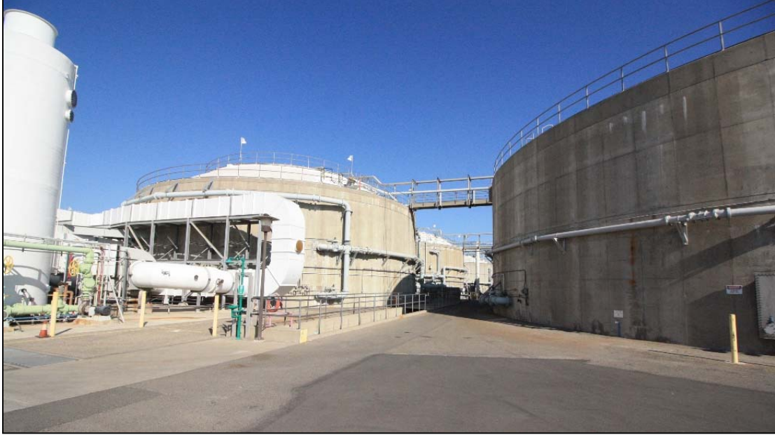
Digesters 7 and 8 near the east boundary of Plant No. 1, view facing north (ESA, 2018)
