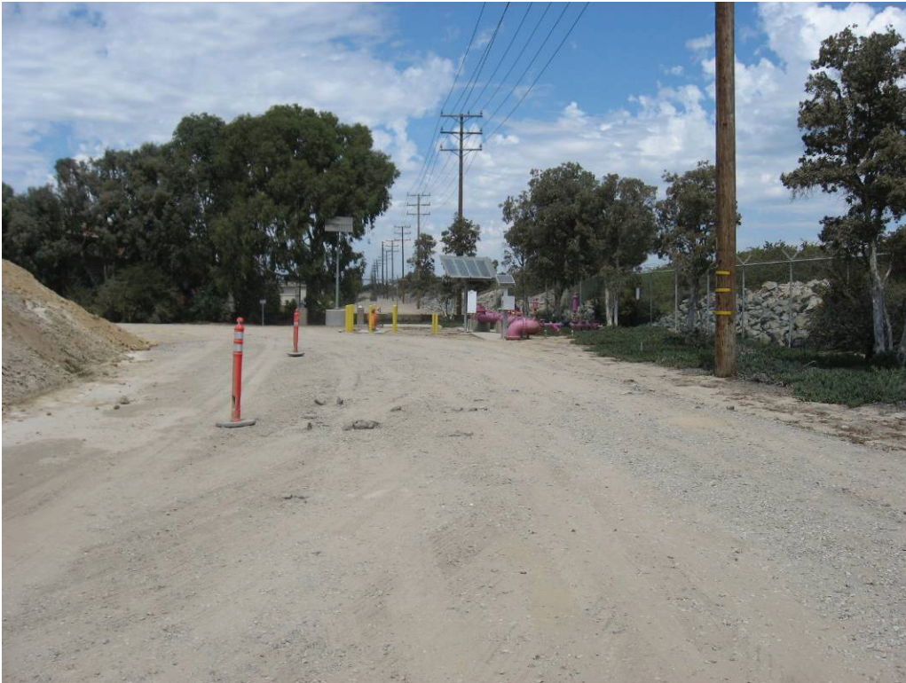
Photo 1: Excavation area and laydown area for OCSD Pipeline (pipeline entry location 1) at the northern portion of the OCSD Plant No. 2 Facility; facing north.
