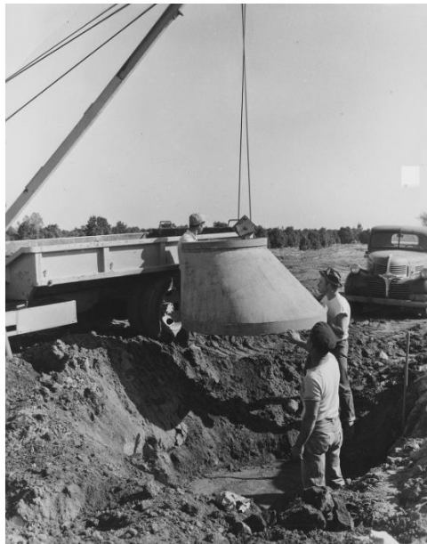
Orange County Sanitation District Plant No. 1 – 150626.00
