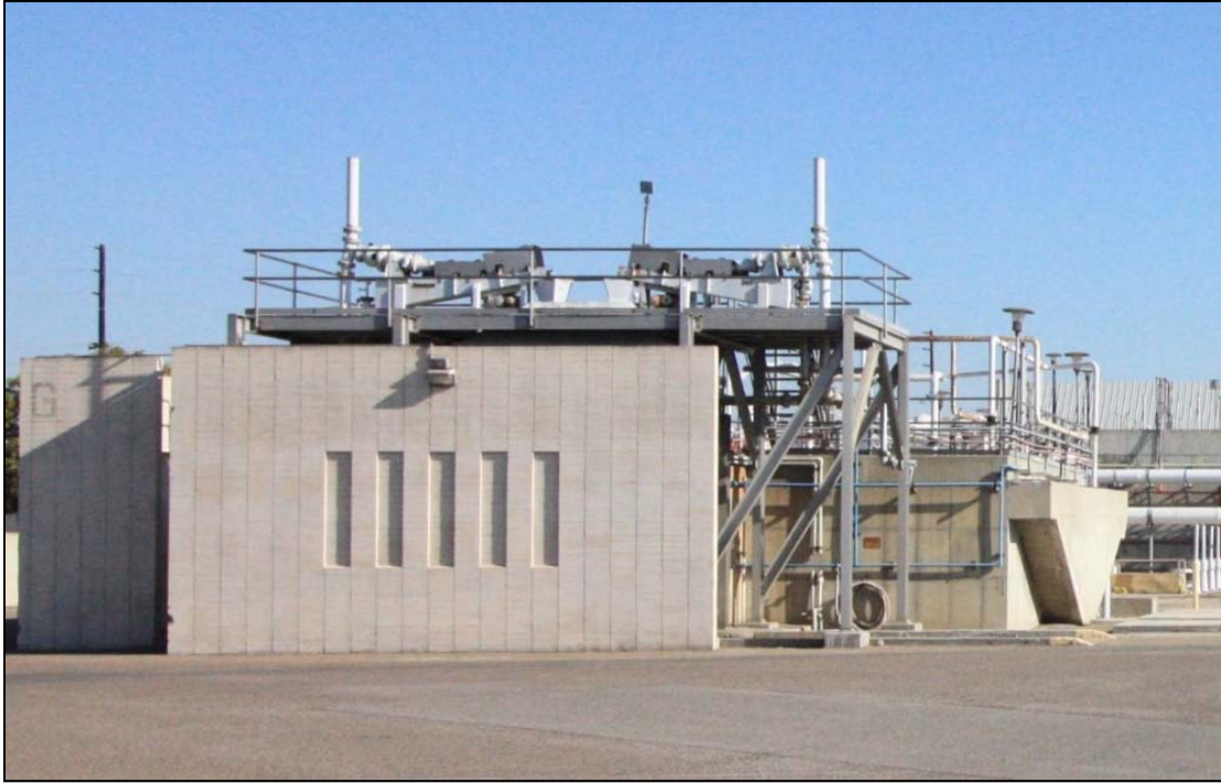
View of Headworks 1, Chlorine Station, and the Grit Chamber, view facing east (ESA, 2018)
